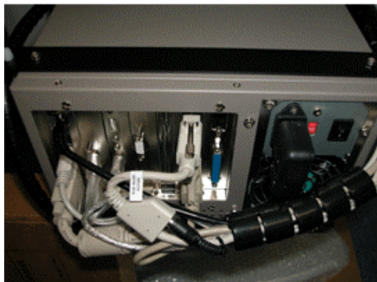
Figure 3: Equipment connections below the PC.
