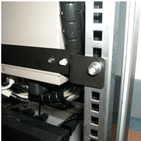
Figure 2: Lower PC bracket attached to the kiosk frame.
